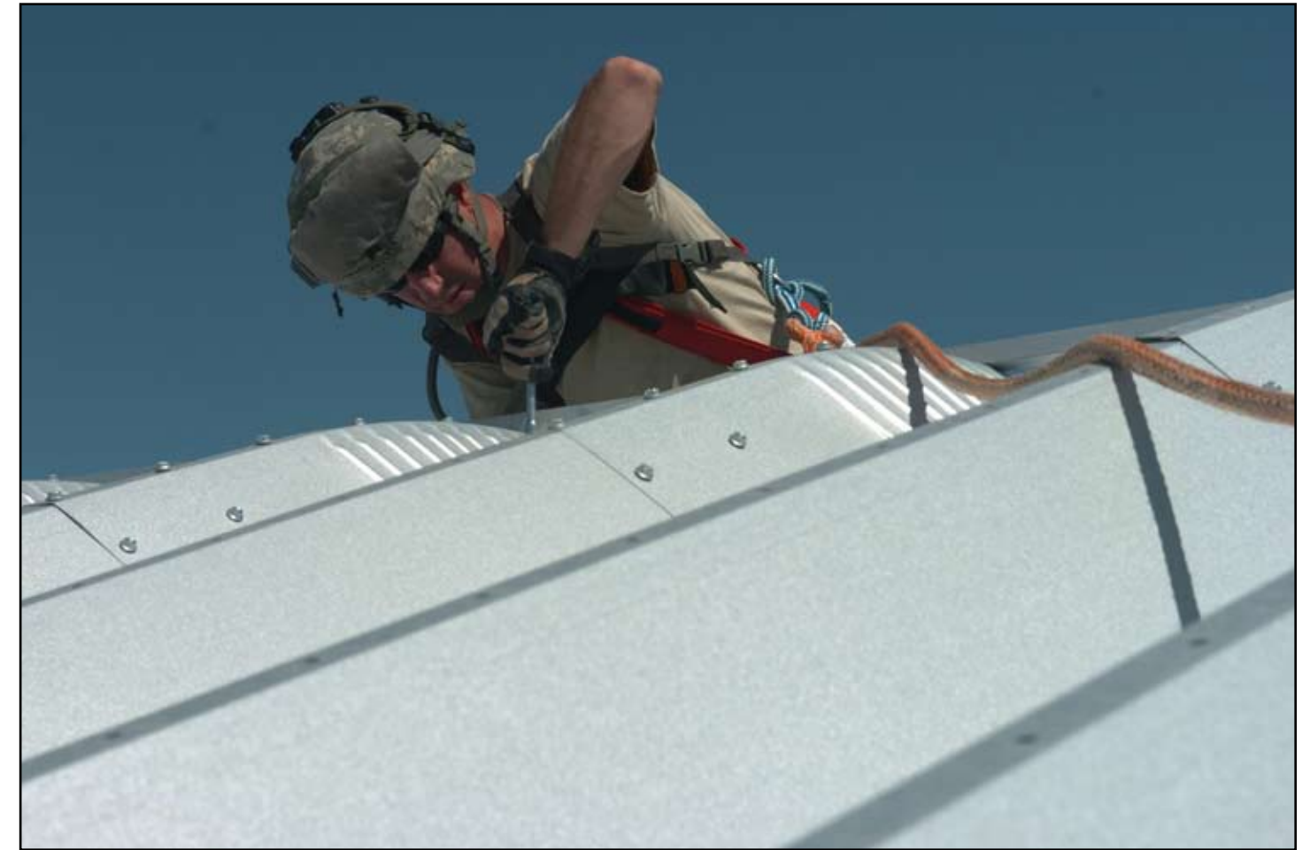
Sgt. Andrew Stang, a carpenter from the 492nd Combat Engineer Company uses a cordless drill to tighten bolts on top of a Quonset hut at FOB Miami during Operation Sand Castle 2009.
