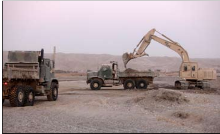
Lance Cpl. Josh Davis, heavy equipment operator, Heavy Equipment Platoon, Support Company, 8th Engineer Support Battalion, 1st Marine Logistics Group (Forward), fills a dump truck while conducting road-improvement operations in Sangin, Afghanistan, Dec. 9.
