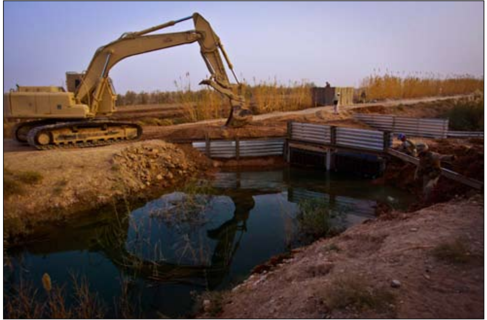
Equipment operated by Marines with Engineer Company, Combat Logistics Battalion 3, 1st Marine Logistics Group (Forward) finalizes construction on a bridge in Marjah, Afghanistan, Dec. 4. Combat engineers with CLB-3 constructed a bridge and guard post in support of Marine units operating in the area.
